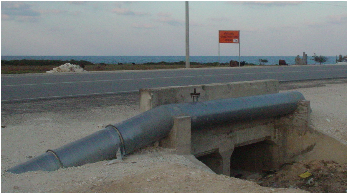
Exhibit 3.7 - Example of Cross culvert with steel pipe (Pictures taken from the Great River-Lucea Water Supply Project)
