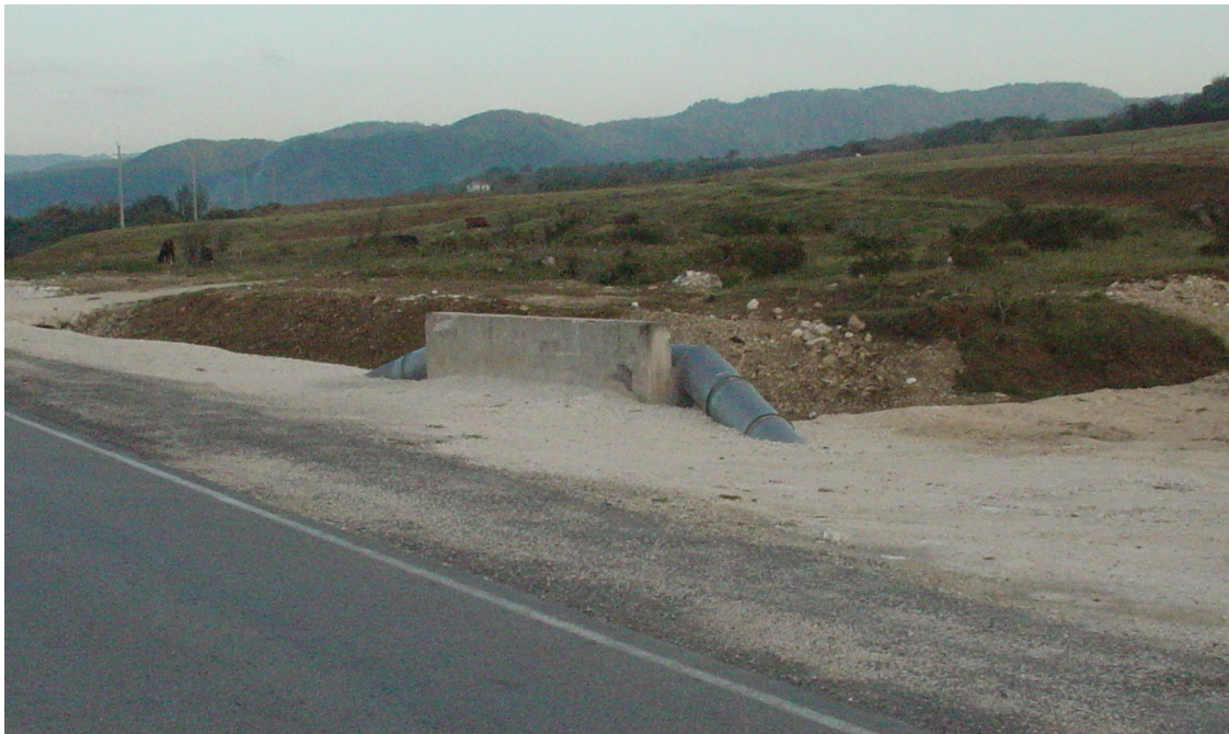
Exhibit 3.6 - Example of Cross culvert with steel pipe (Pictures taken from the Great River-Lucea Water Supply Project)
