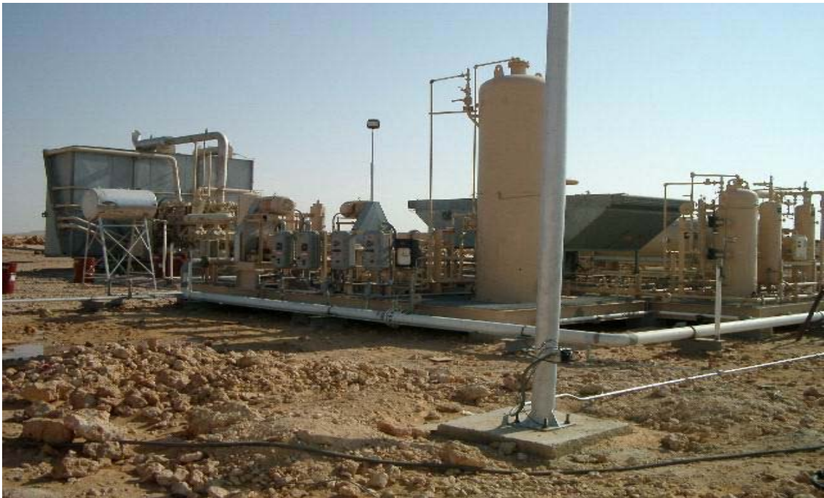
Nodal Compressor Station (Khalda)
