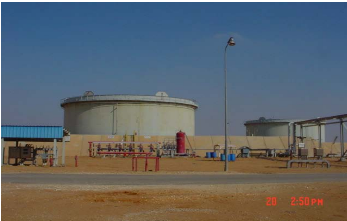
Storage Tanks – Qarun Oil Process Facility
