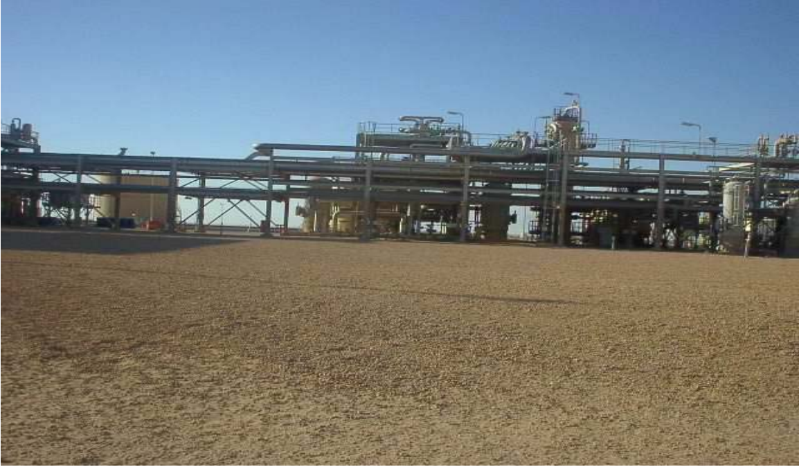
Salam Gas Plant (Khalda)
