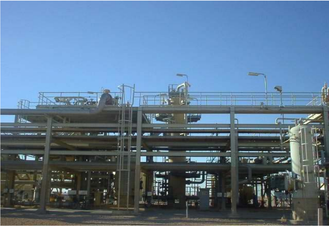
Salam Gas Plant (Khalda)
