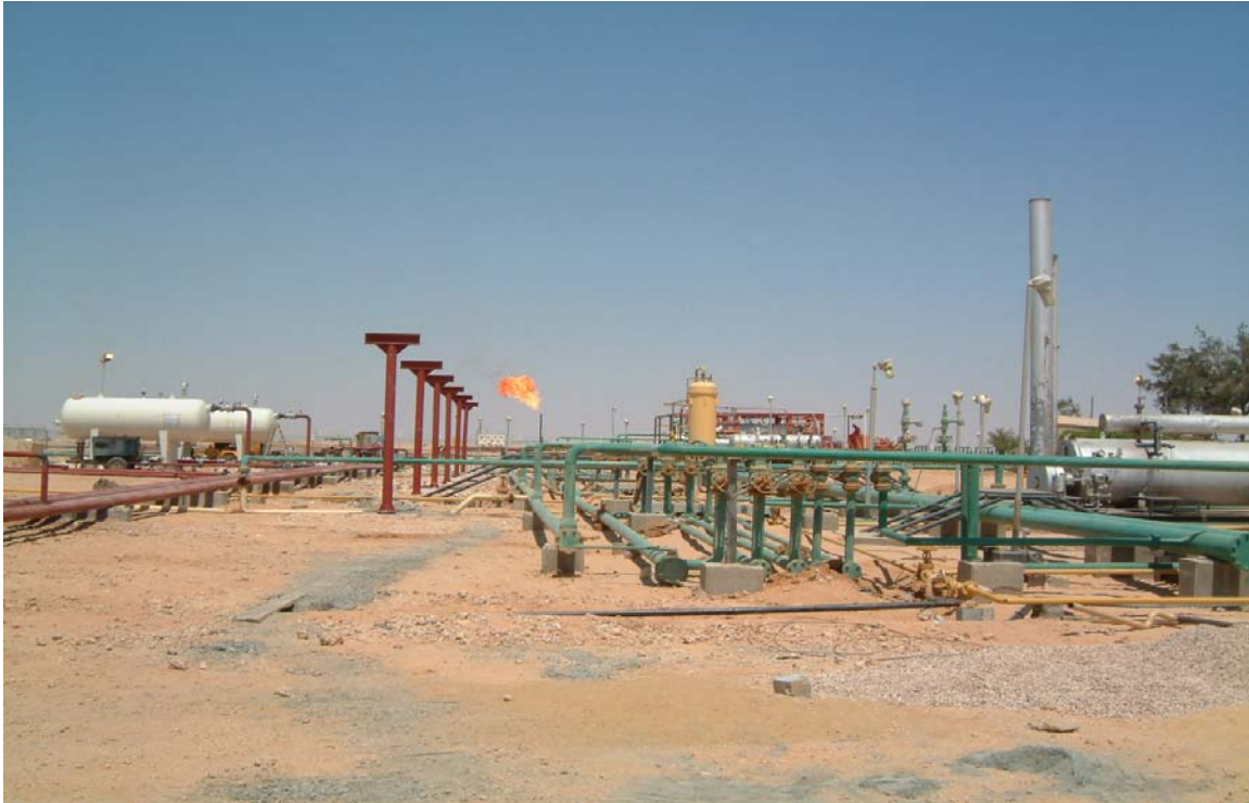
Umbarka Process Facility
