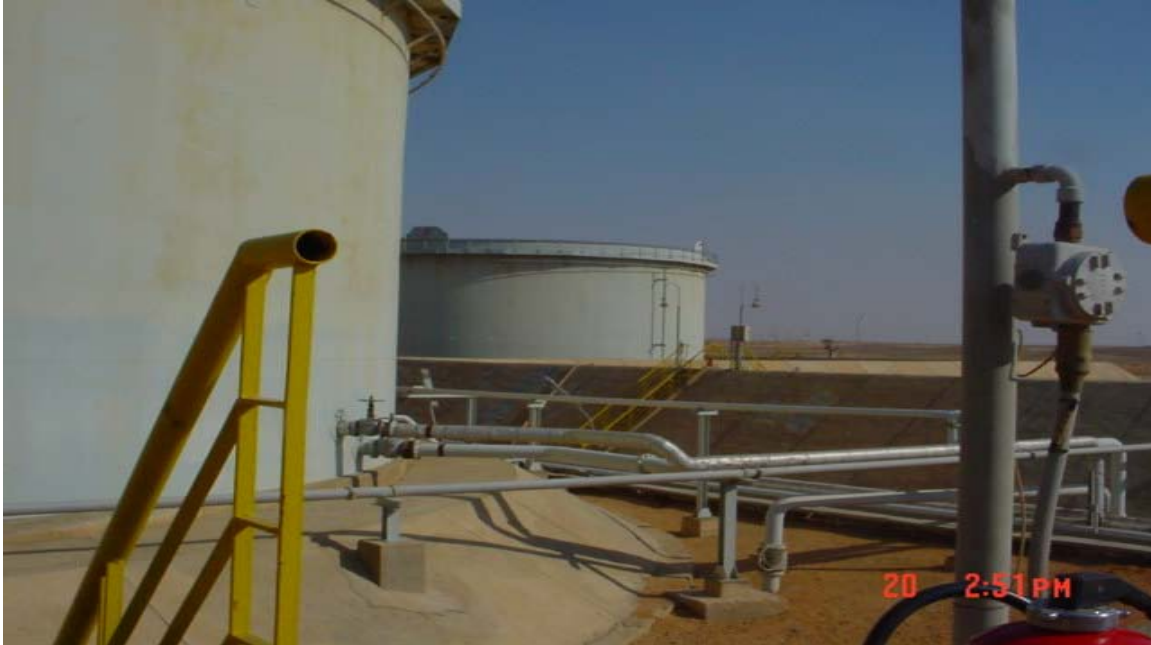
Tank Containment - Qarun Oil Process Facility
