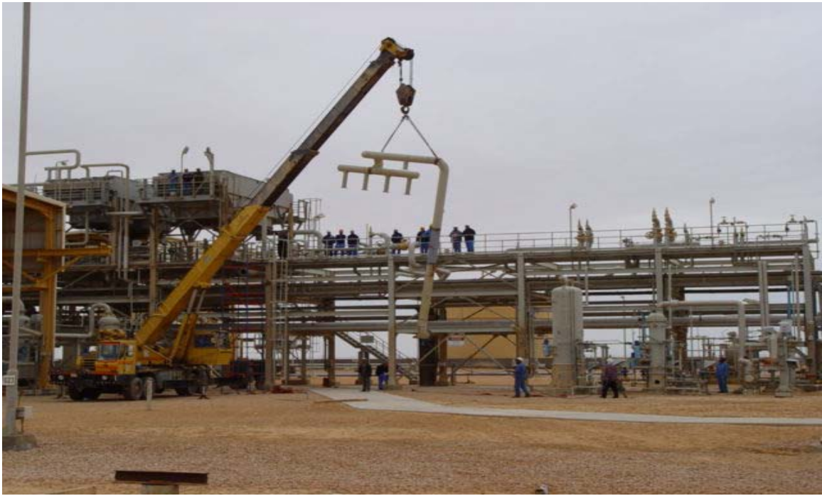
Tarek Gas Plant (Khalda)
