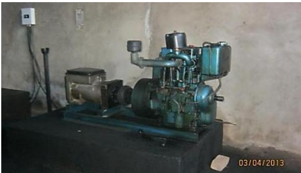
Figure 23: Diesel Generator at the Ranch
